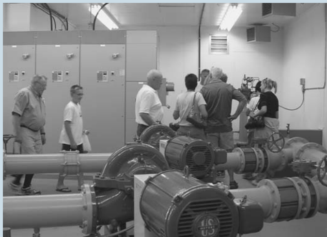
Union Road pump station.
